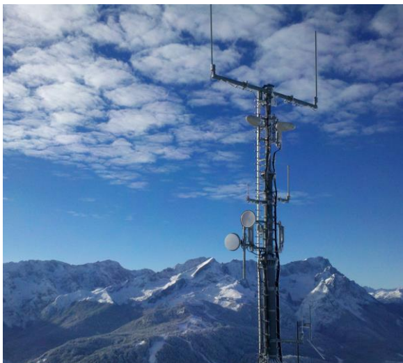
From radiation differences between transmission masts of mobile network operators, meteorologists can derive information on rainfalls. (Photo: Christian Chwala)
